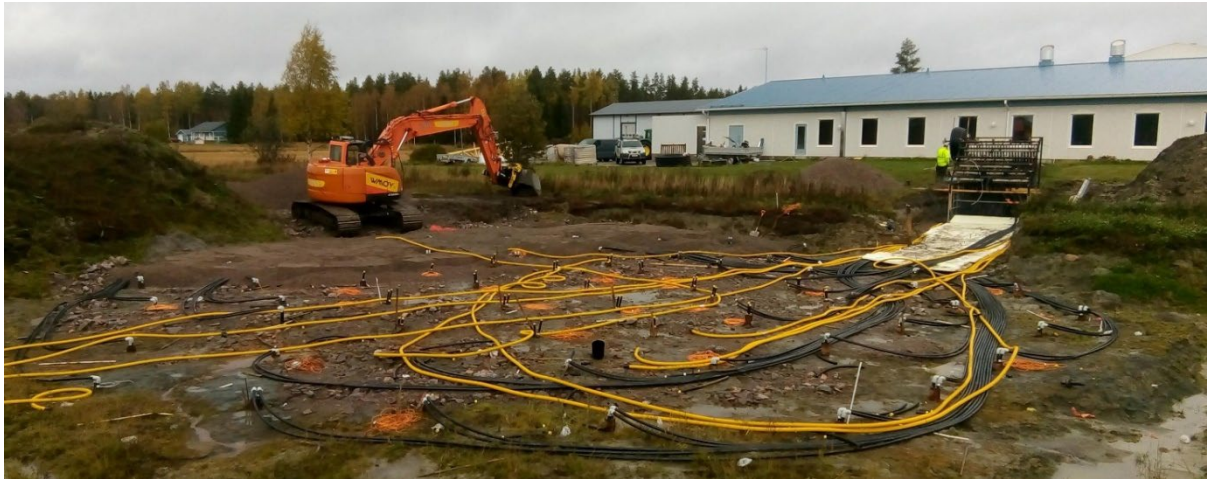
View of the borehole thermal energy storage during the construction phase at the Finn Spring factory.
